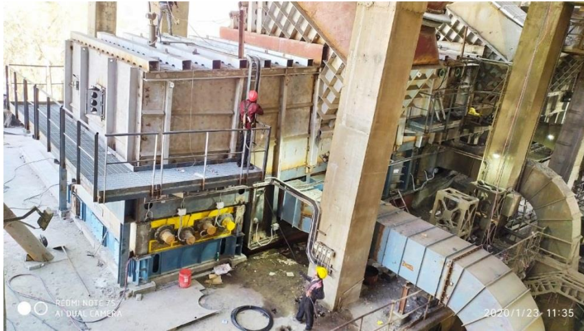
Top view of extended part of Clinker Cooler
